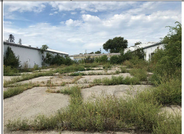
View facing north of former floor slab for one of the oldest site buildings.
