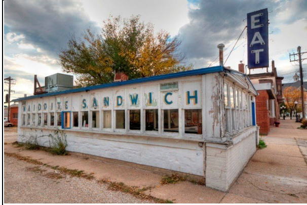
View of former Maid Rite Sandwich Shop in Macomb in 2007 (original photo by Robert Lawton) 1
