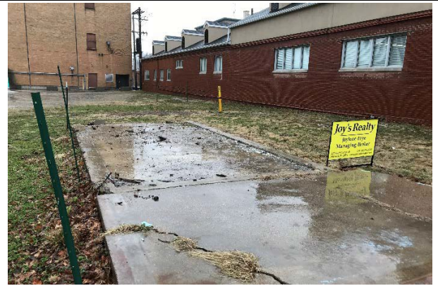
View facing SW of Main Parcel in 2020 with former restaurant floor slab in foreground.
