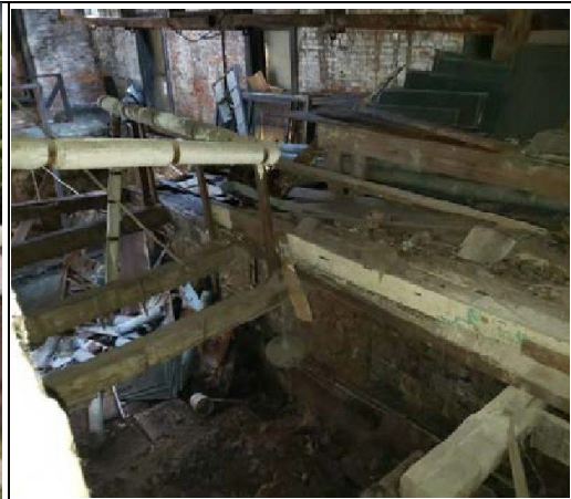
Collapsed floor in interior of rear building.
