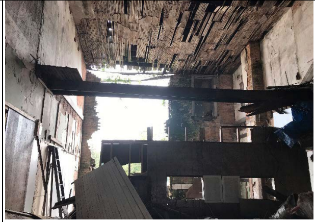
View of the interior of one of the buildings showing the partially collapsed rear wall.
